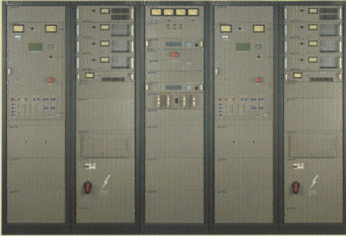
Armstrong 60000 Watt FM Transmitter System
